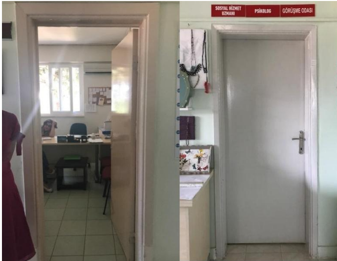
Figure 9. Insufficient door widths (Mersin and Tarsus CMHC)
